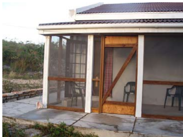
Residential side of the building, with its new insect screening. Part of the new wall to deflect water and mud slides is visible on the left.
