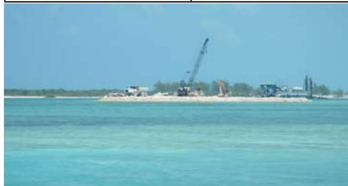
Artificial island being created by pumping dredgings on to the sea-grass beds in the Princess Alexandra National Park, adjacent to the Nature Reserve islands (behind workings and out of view near camera position).
